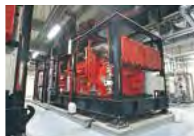
Reducing CO 2 emissions with a highly efficient cogeneration system.
