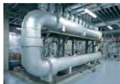
This heat exchange system cools our injection molding equipment with heat from an electrical generator.
